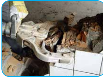
HCS 8 B replaces the sledge hammer to break down brick wall 32cm
